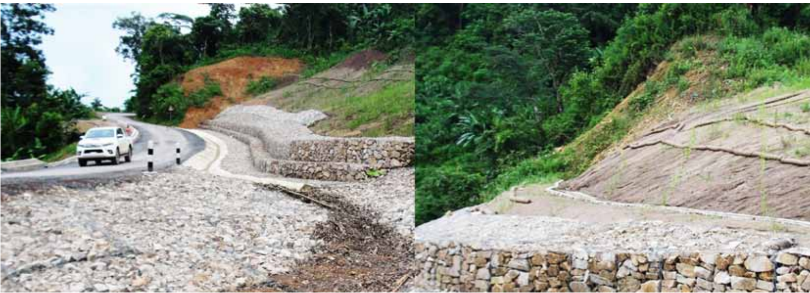
Slope stabilization structures were completed along key roads in Bountai District, Phongsaly Province
