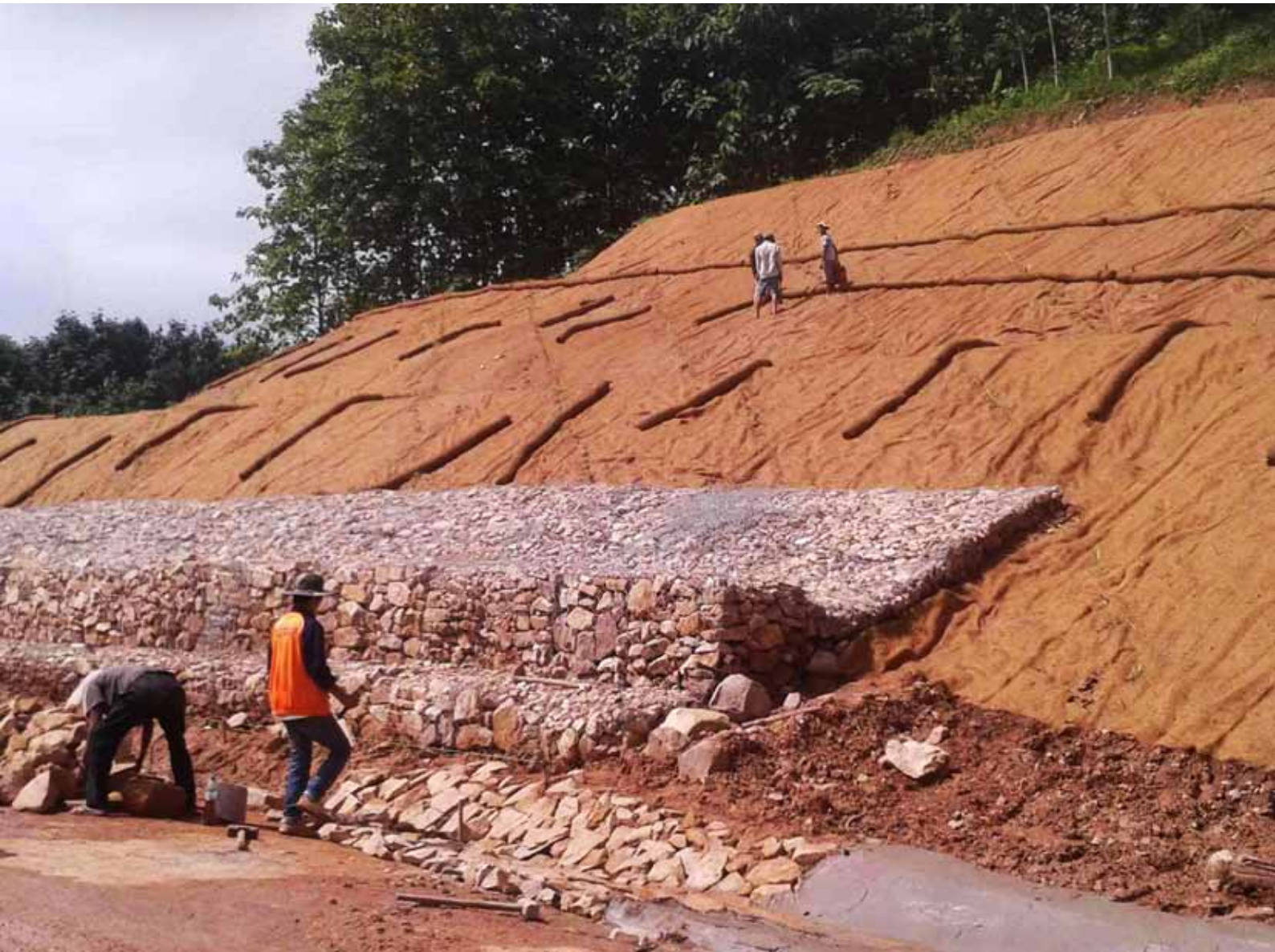
Safe road construction, including the installation of slope stabilization structures, was a key part of providing safer community infrastructure in risk prone locations
