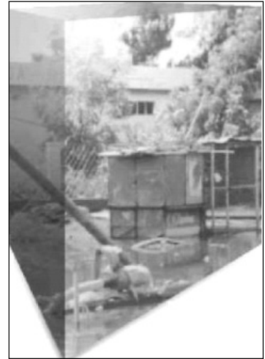
One of the drainage system's pumping stations underwater
