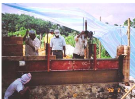
Cost-effective construction activities on Relocated Land using slip-form technology and a low cost material mix of soil and cement
