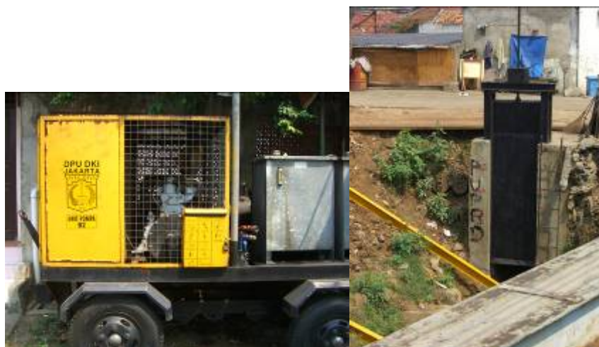
Figure 7. Pumps and Gates in Kebon Baru Area
