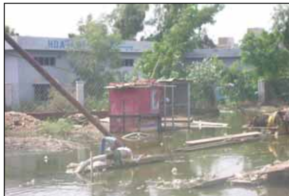
Pumping station is submerged under rainwater
