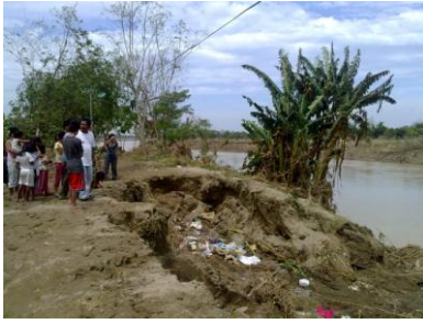
Riverbank erosion in Dagupan after Typhoon Parma
