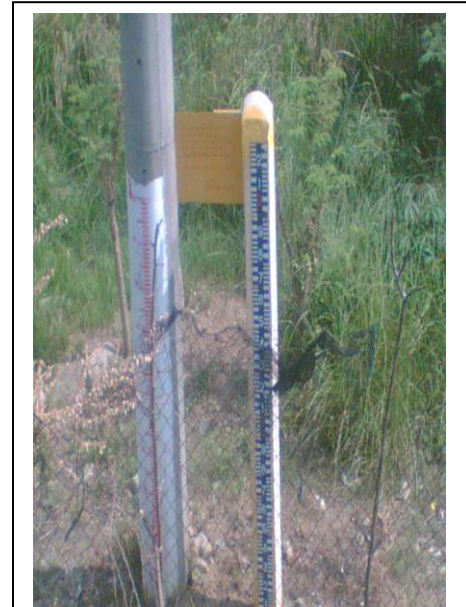
A device used to measure the water level during typhoons or high tide
