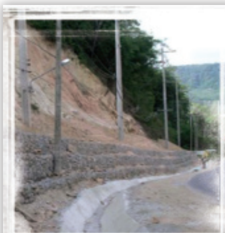
Gabions, cages filled with rocks, sand or soil, help to stabilize the slope from erosion. Image credit: RECLAIM
