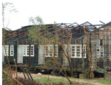
Roof-top remained concern for most of the houses
