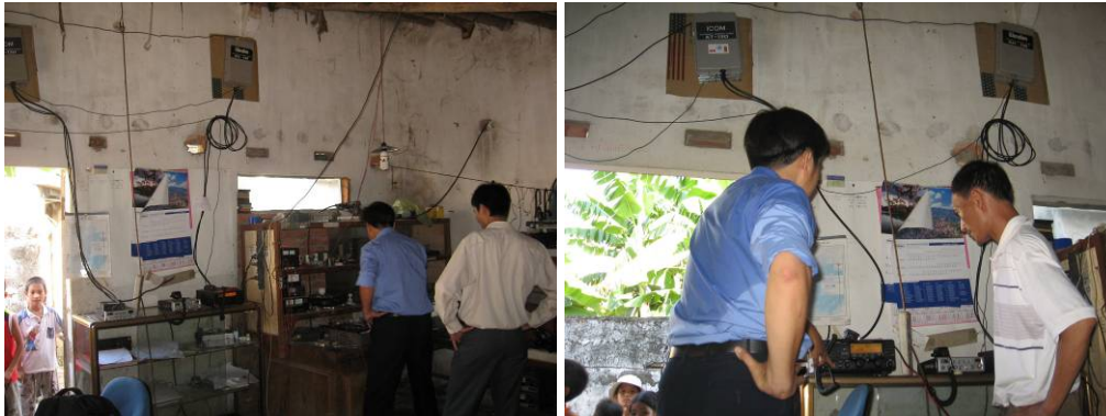
Upgrading the ICOM equipment and operations of Ngu Loc commune early warning center in Thanh Hoa province, Vietnam
