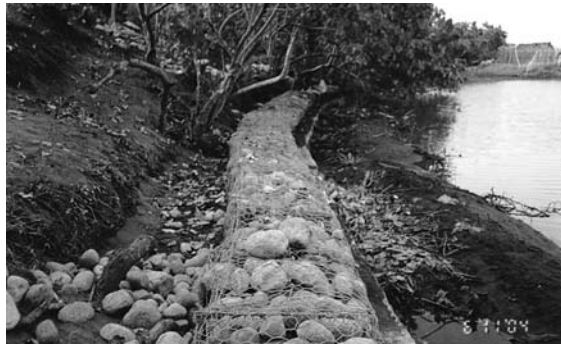
Diversion Canal in Municipality of Sagnay, Camarines Sur constructed during the DIPECHO Project with Spanish Red Cross support.
