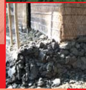
Raising of plinth, one of the structural mitigation needs that the communities identified during the VCA process.
