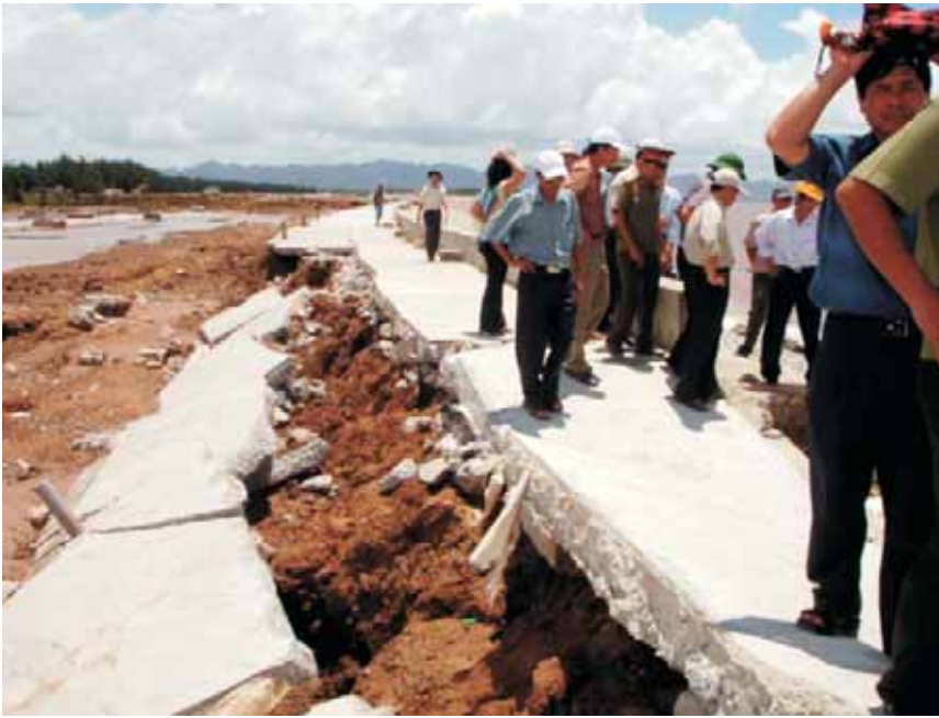
Damage caused by the Damrey Typhoon in July 2005 to Hai Hau in Nam Dinh Province.
