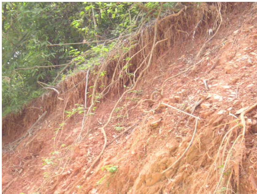
Figure 10. Slope degradation due to weak vegetation cover.
